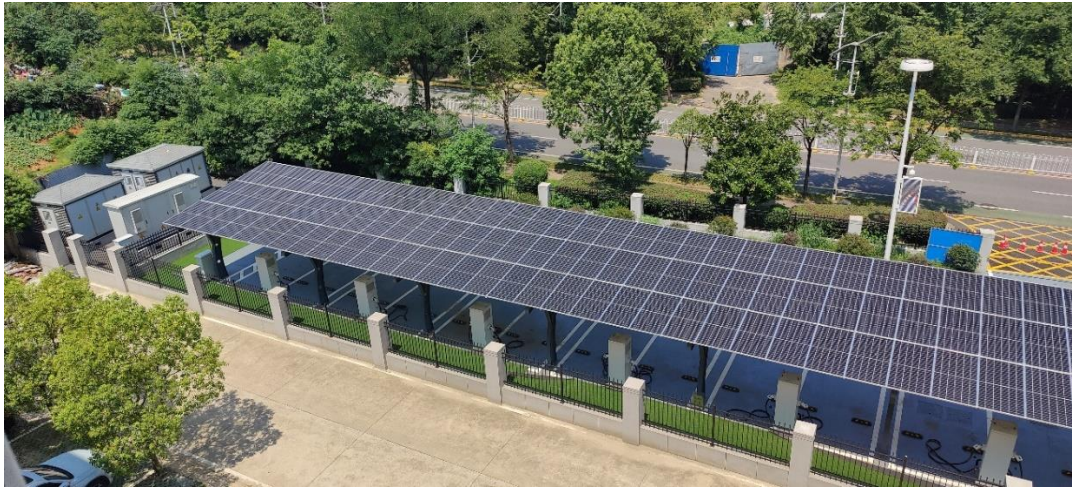
Figure 17 Photovoltaic site photo of metal processing factory case
